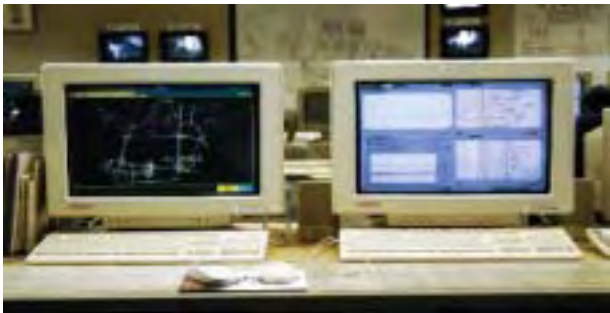
Centralized monitoring computers
